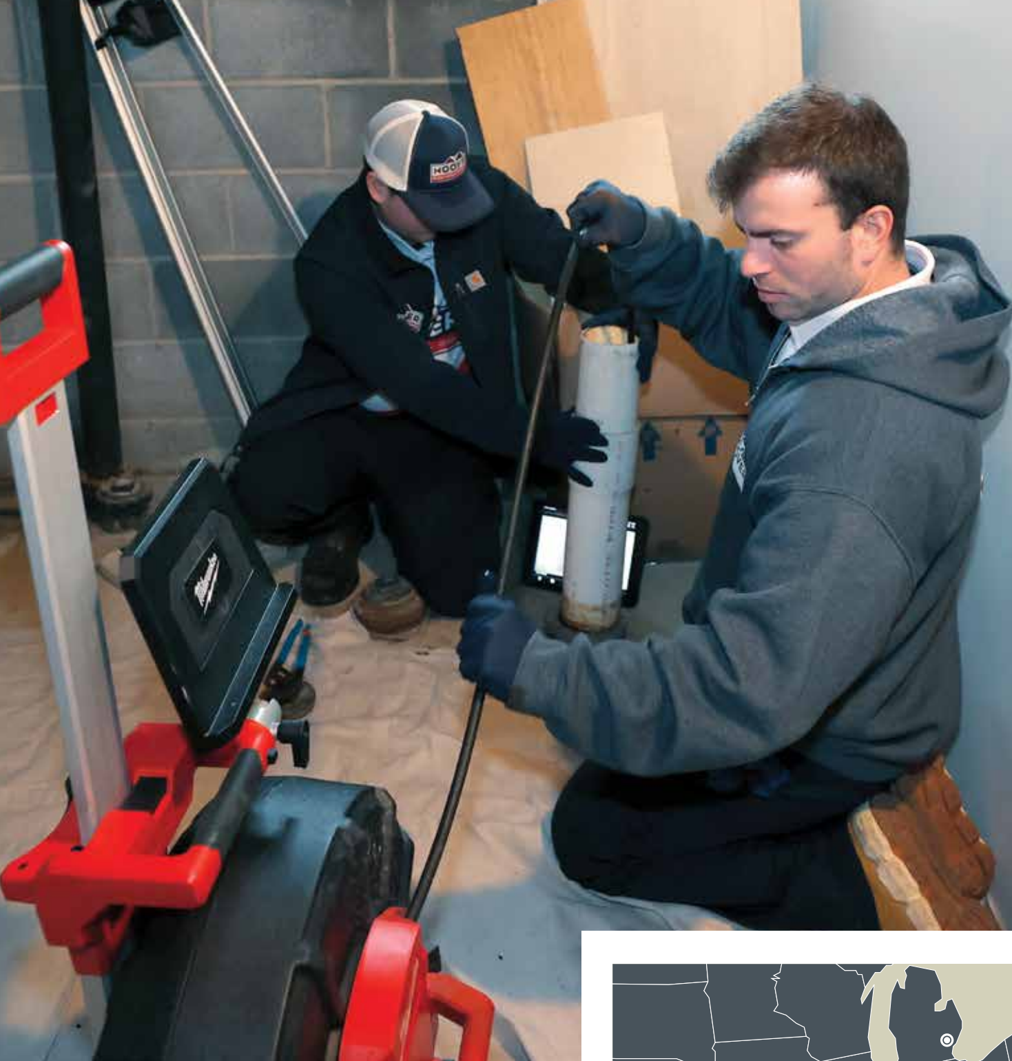
« Connor Murphy and Trevor Gilbert use an M18 series inspection camera from Milwaukee Tool on a residential job in Oak Park, Michigan.
