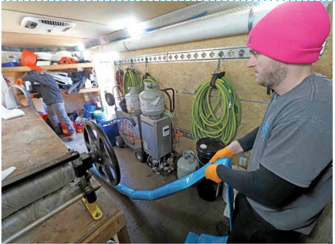
Lead CIPP technician Greg Simon (right) wets out a liner in one of Marvel's operations trailers as Garvey assists him.
