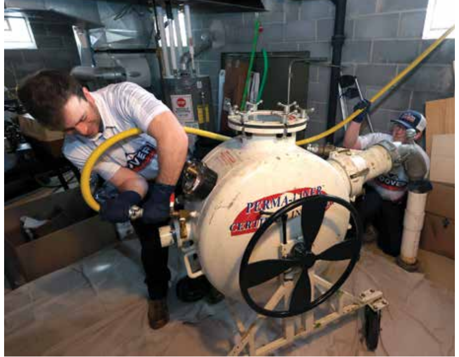
▲ Gilbert attaches an air hose to a Perma-Liner system before beginning work on a liner installation.
